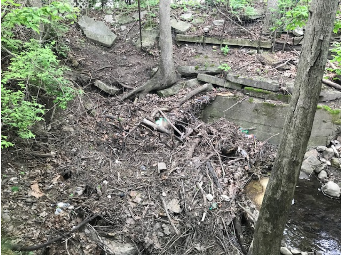
Ess Creek Photo 3: Existing Ess Creek headwall's wing can be seen. The inlet to the Ess Creek Storm Sewer is buried by the debris.
