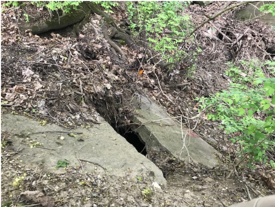
Ess Creek Photo 1: Large concrete slabs, with eroded voids in the bank underneath, cover the private storm outfall from the church parking lot north of the project site.
