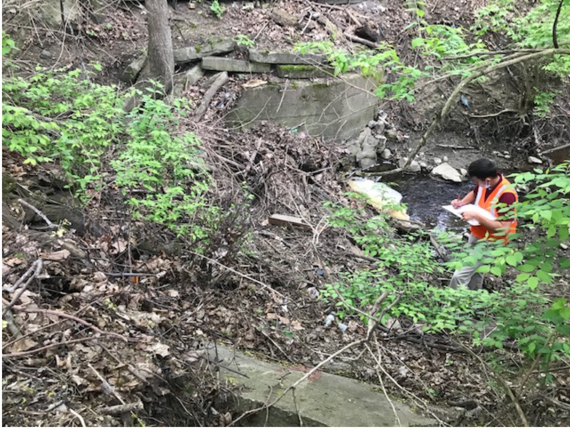
Ess Creek Photo 2: Concrete slabs from Photo 1 are shown along with the existing Ess Creek headwall's wing in the background.
